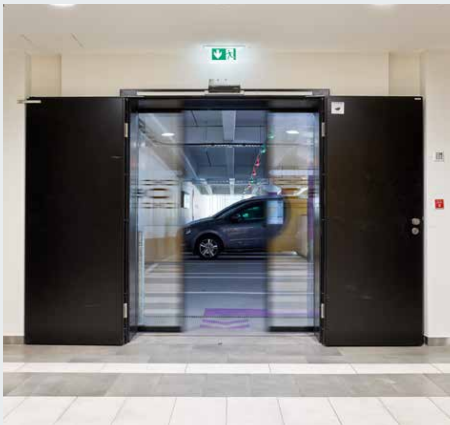
Viewed side of fire-rated and smoke-tight door (daytime operation)
